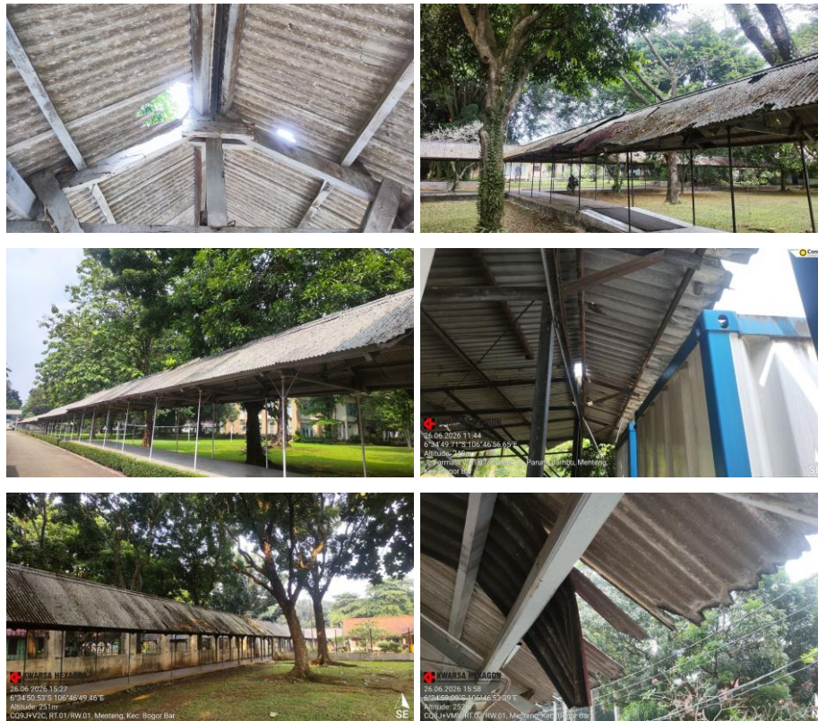
Figure 14.2. Asbestos Containing Material Identified During Visual Survey
